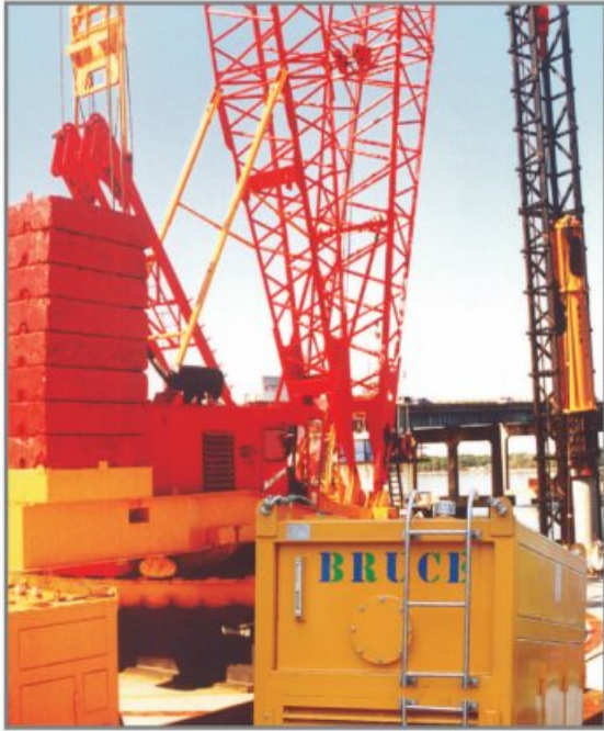
BRUCE SGH-3013 working at bridge foundation site at Panama City, Florida, USA driving concrete pile (O.D 60" x I.D 45" x 120 feet long)
