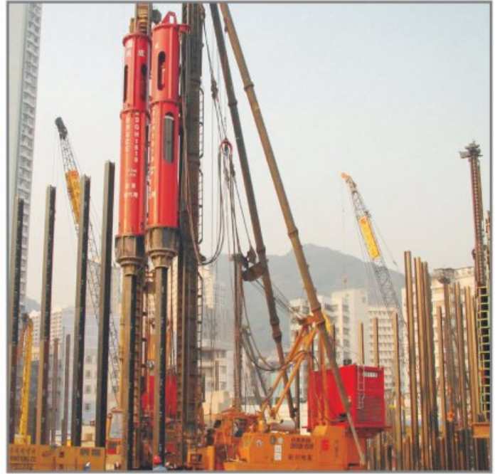
BRUCE SGH-1618 & 1619 at Hong Kong driving H-beam piles (305mmx 305mm, 223kg/m, 48m long)
